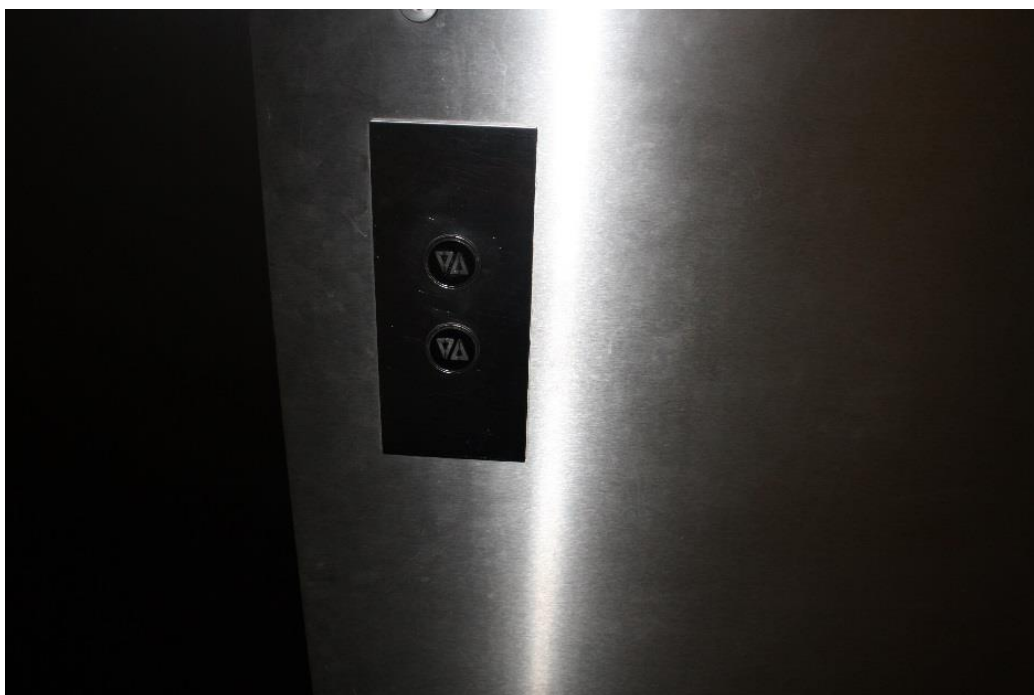
Image 4: This is a photograph of the buttons used for calling the lift. The circle and arrows are slightly raised, they also light up red when pressed.
